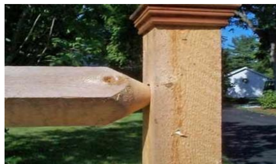
Figure 19. Dowel Joint (not acceptable)
