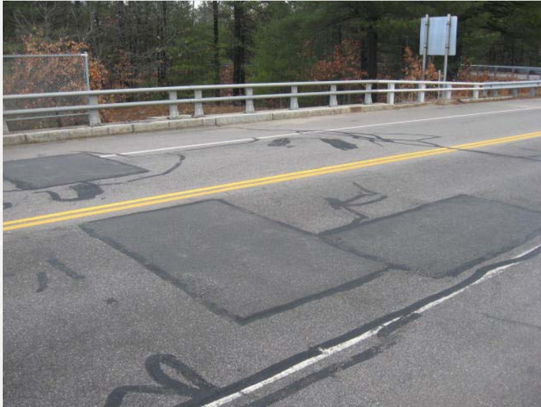
Patched areas on surface of bridge deck
