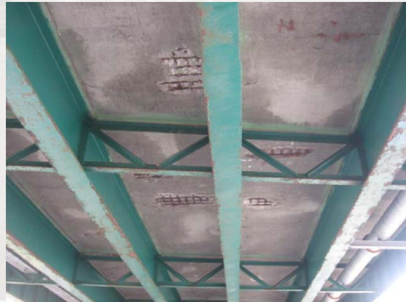
Concrete delaminations on underside of bridge deck
