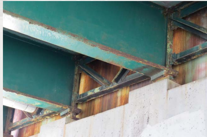
Paint failing – rust staining
